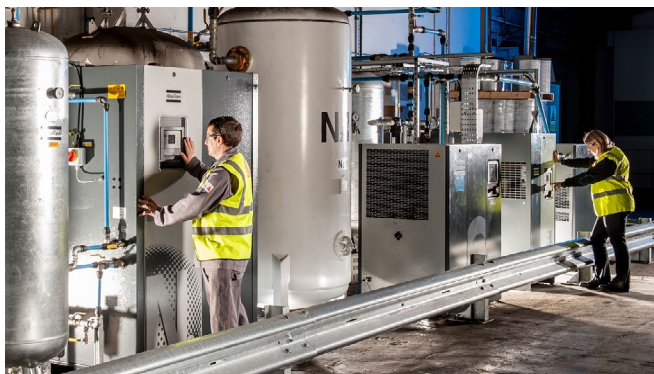
Three GA compressors provide dry compressed air and two NGP units provide nitrogen for batch mixing and for topping off containers
