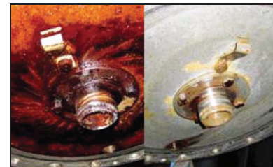
Vessel cover contaminated
