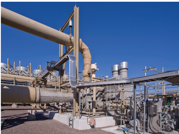
Generating electricity from geothermal heat.
