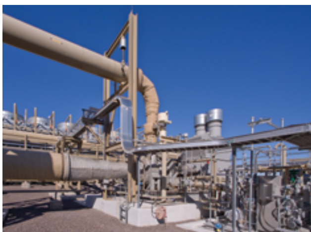
Generating electricity from geothermal heat.
