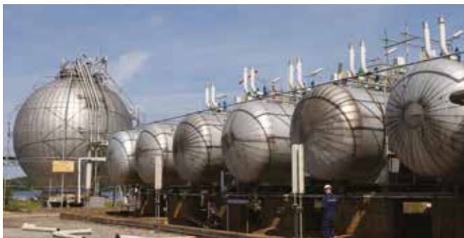
Inside an ethylene-oxide plant
