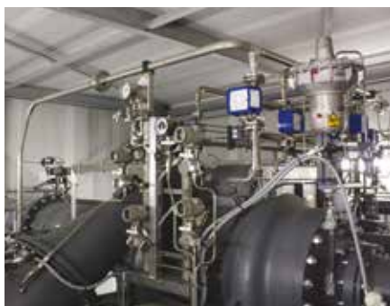
CO 2 gas compressors are used in pipeline applications.
